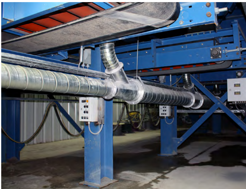
Fugitive silica dust, generated as material is poured into storage silos, is captured at the source and conveyed to an outdoor dust collector through this ductwork system.
