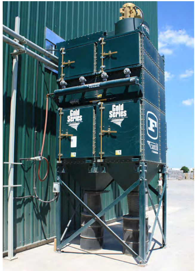
High efficiency cartridge dust collector contains fugitive silica dust at a batching plant used in the manufacture of paving stones.
