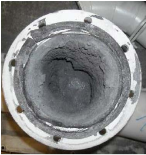
Figure 6 – Clogged ductwork conditions caused by inadequate filtration
